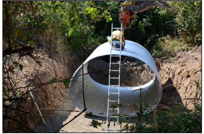
Construction in 2017 to replace a North Fork Johnson Creek culvert under the Springwater Trail. This is the lowest downstream location of 7 culverts being replaced, removed or retrofitted to provide fish passage on this tributary. Construction activities are phased over a three year period, 2016-2019. Source: Daniel Newberry, Johnson Creek Watershed Council
