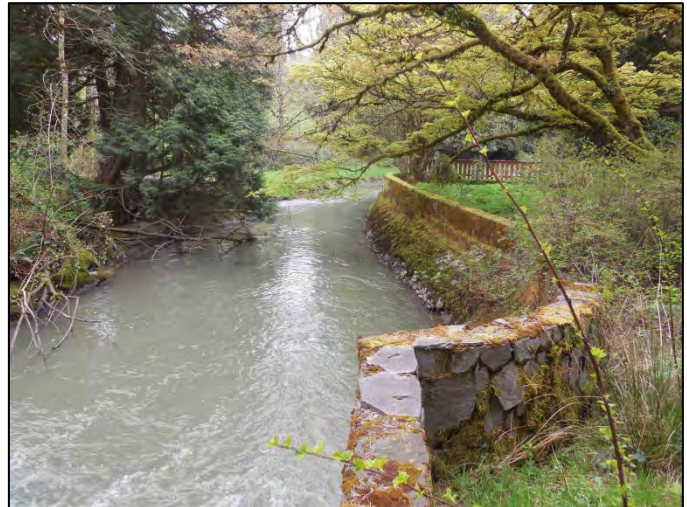
A retaining wall along upper Johnson Creek on Metro’s Ambleside property. Planned restoration will remove the streamside walls, demolish a concrete weir, and add large wood jams throughout the reach to improve channel and floodplain function. Source: Brian Vaughn, Metro
