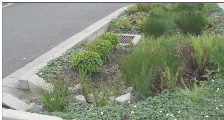
A curb bump-out and rain garden in Portland, OR. Photo: DC Green Infrastructure
