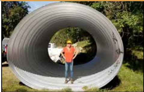
The new culvert has a natural stream bottom and opens access to a half mile of spawning habitat.
