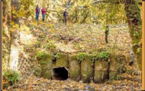
Perched and failing culvert blocked fish passage in this essential habitat stream.
