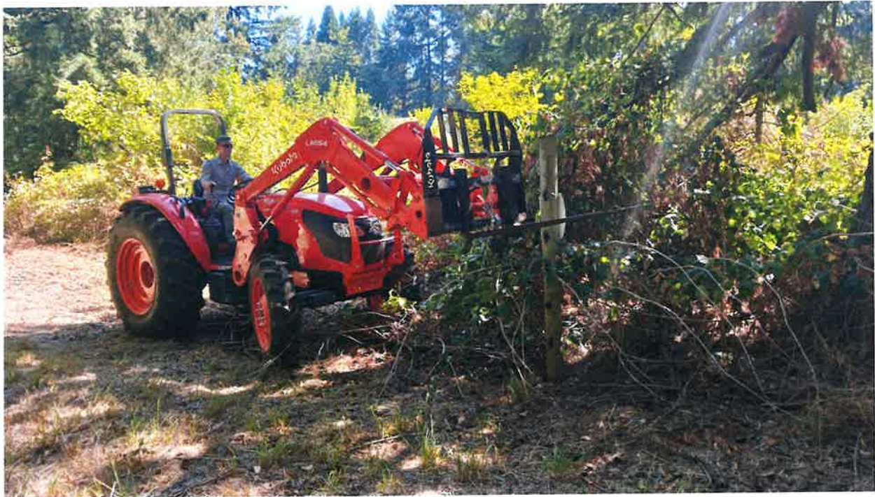
Figure 4 - Gus pulling posts from the south fence line in preparation for replacement
