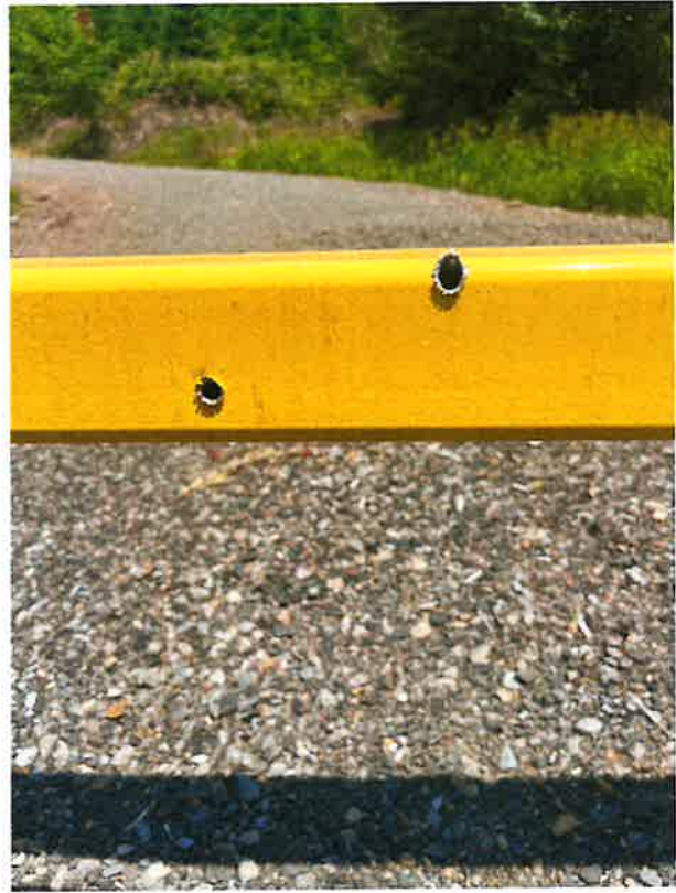
Figure 3 - Gate damage from unauthorized firearm use
