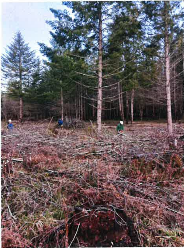
Restoration contractor crew cutting and piling debris at Horner Road site to prepare for reforestation.
