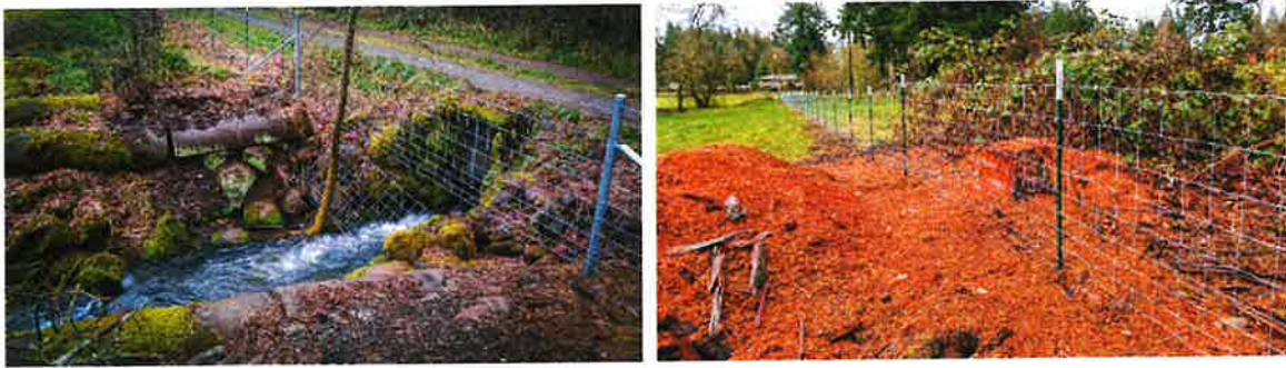
Figure 4 - Stream spanning of the new fence on left, stump removal in fence line on right
