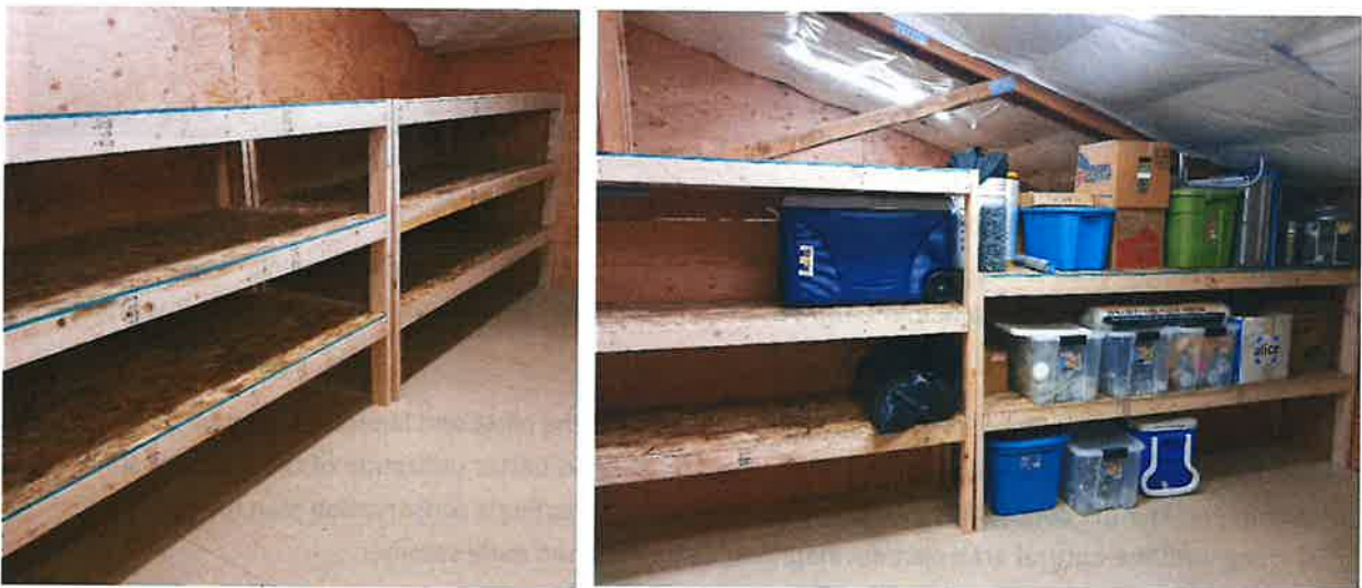
Figure 1 - Archival file shelves are shown on the left with other shelving shown on the right
